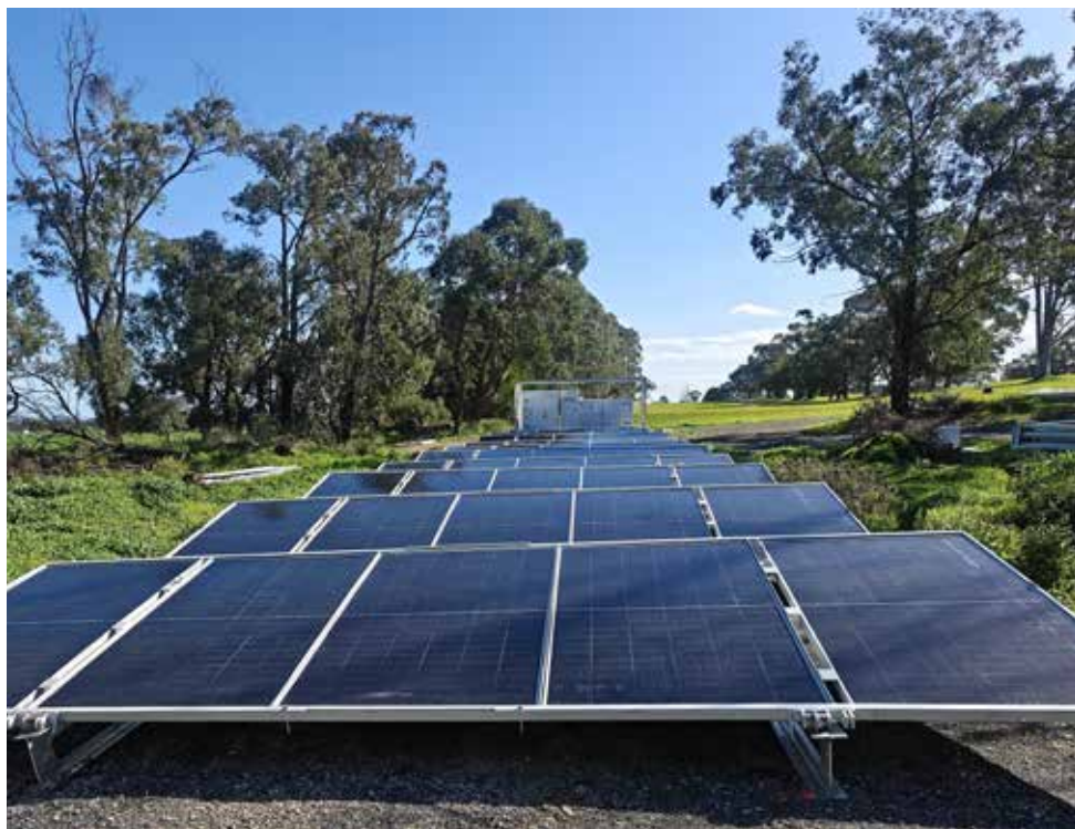
Trafalgar Golf Club's 35kW solar panels
