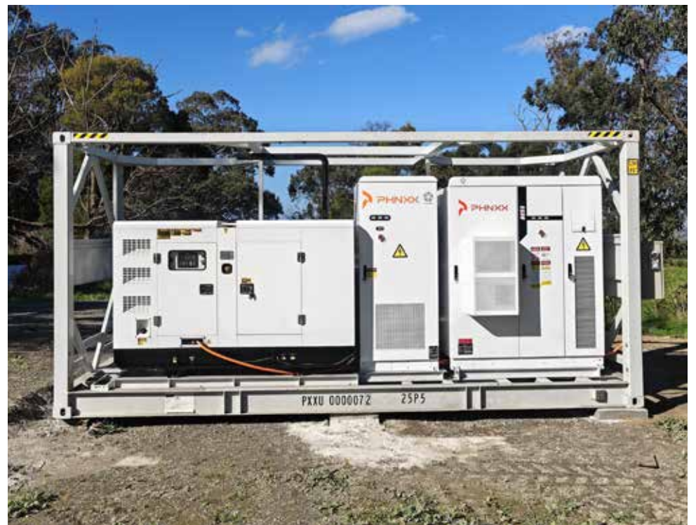
Battery and generator at Trafalgar Golf Club
