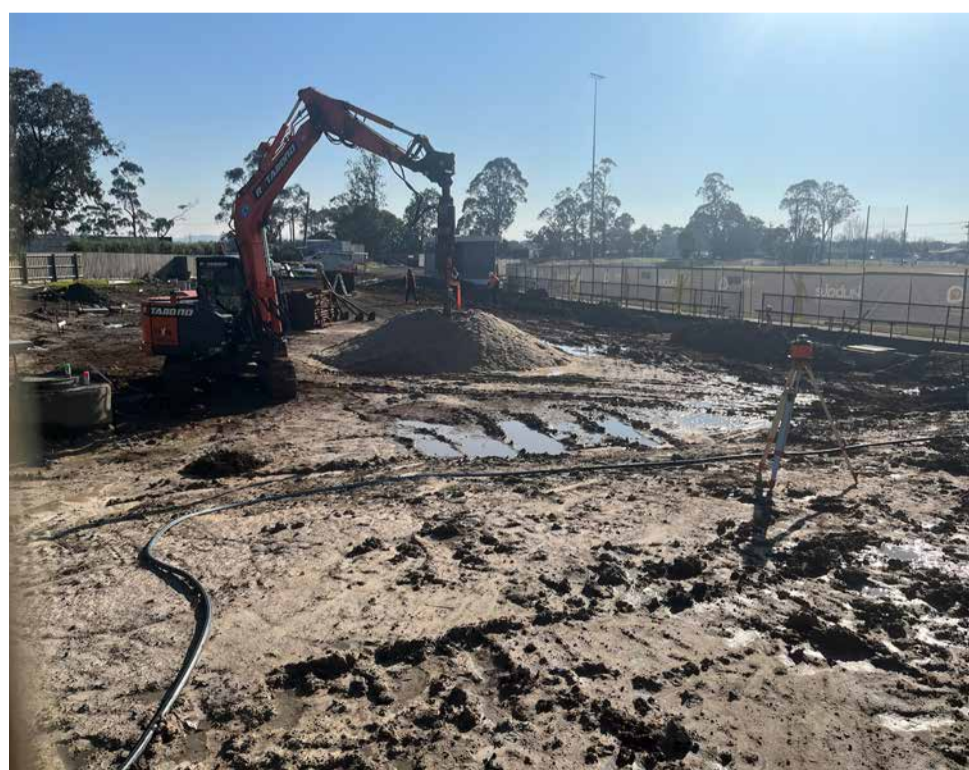
Works begin on the new Downton Park clubrooms in July last year
