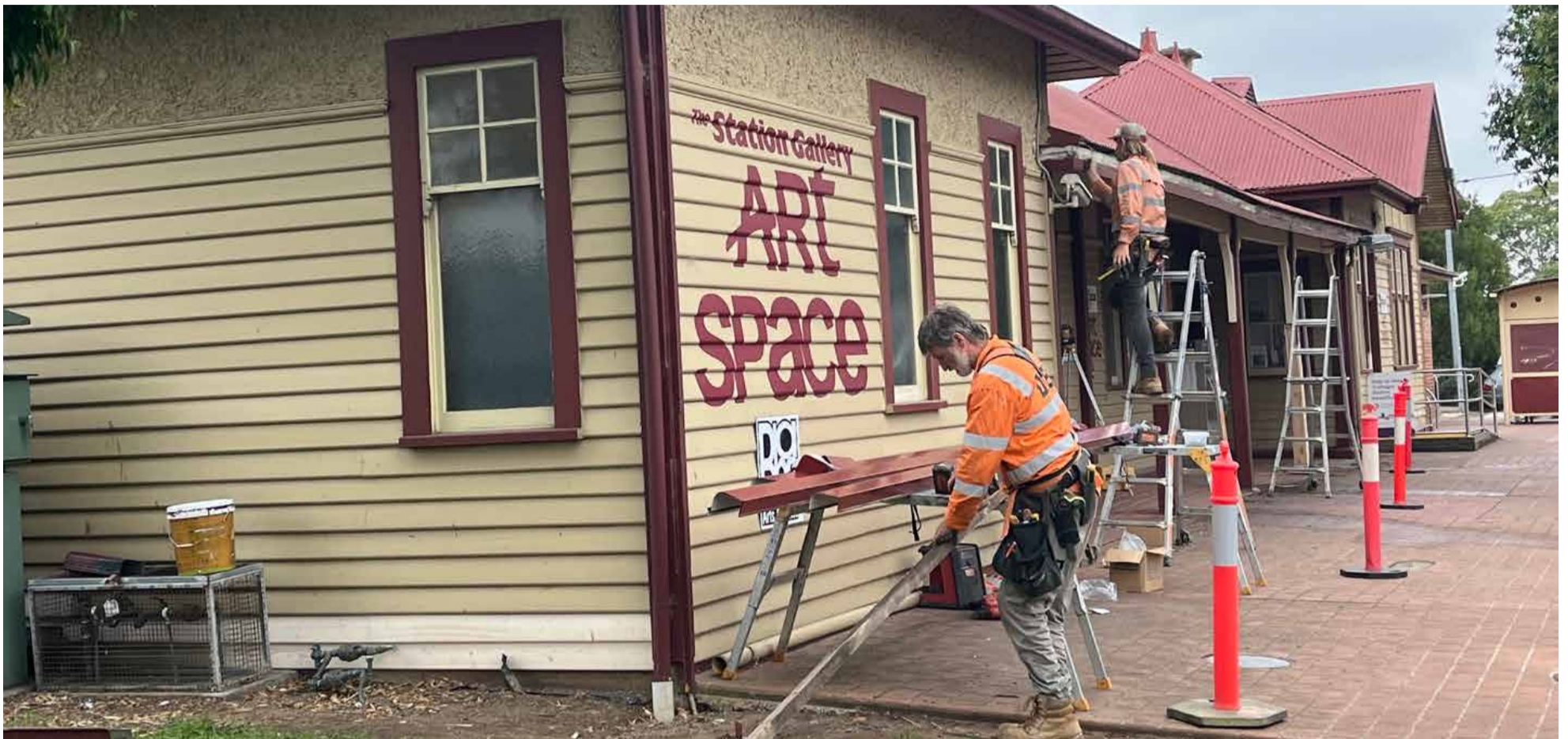
Workers from Direct Property Building Services replacing weatherboards and window frames on Trafalgar Railway Station's building as part of larger maintenance works.
